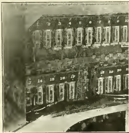
FIG. 17. BANK OF SWITCHES OR CONTACTORS.
